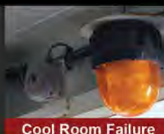
Cool Room Failure
