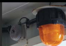
Cool Room Failure
